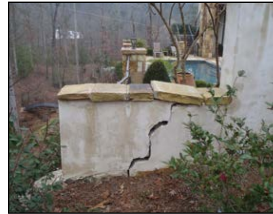
ABOVE: the settling foundation led to cracks in the retaining walls
